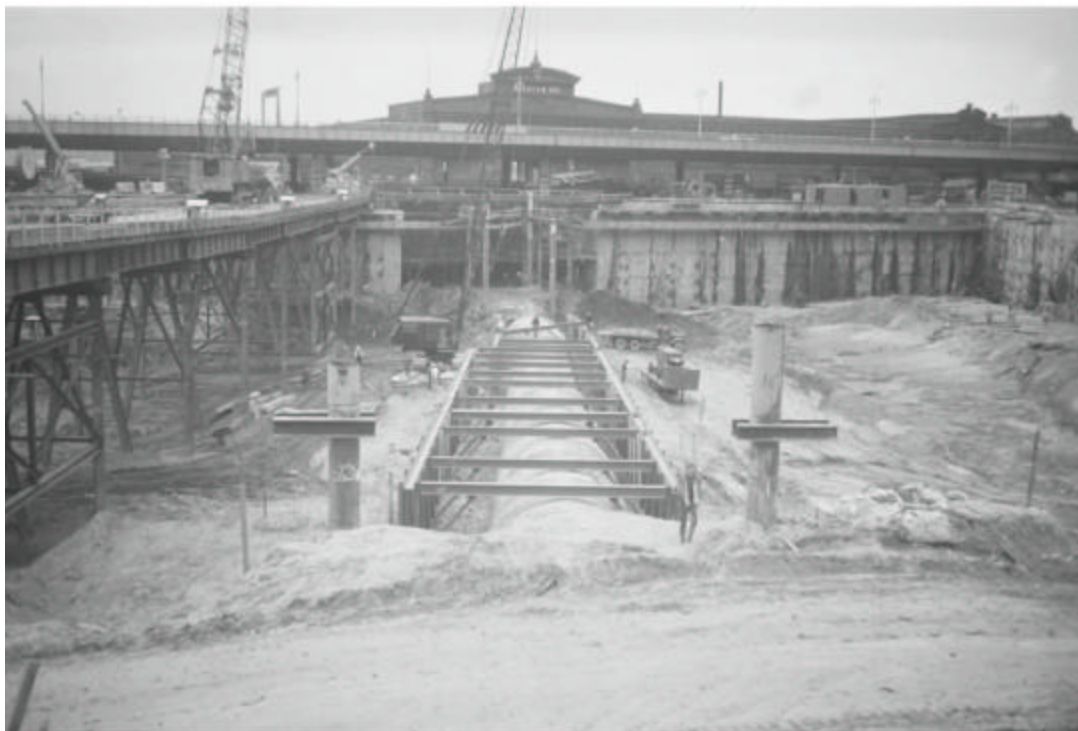
PATH Tube Saddles supported by truss, steel straps between saddles
