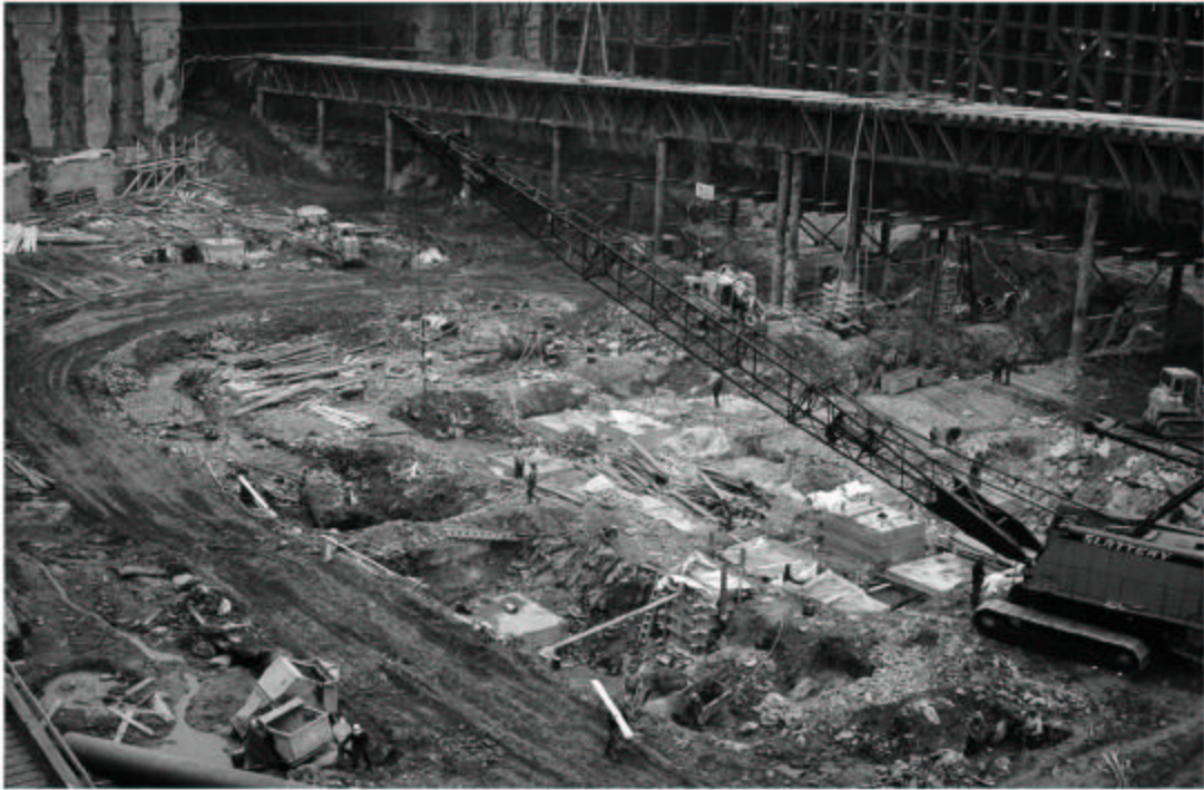
Steel grillages being constructed for North Tower adjacent to supported North PATH Tube
