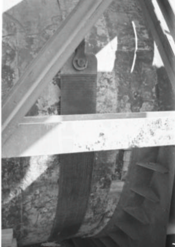
Steel Strap Supporting Path Tube
