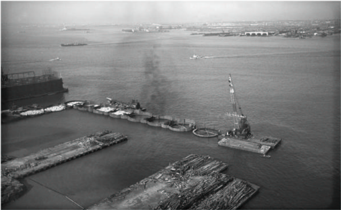
Cofferdams, piers to be demolished, (South West area at different stages of construction)
