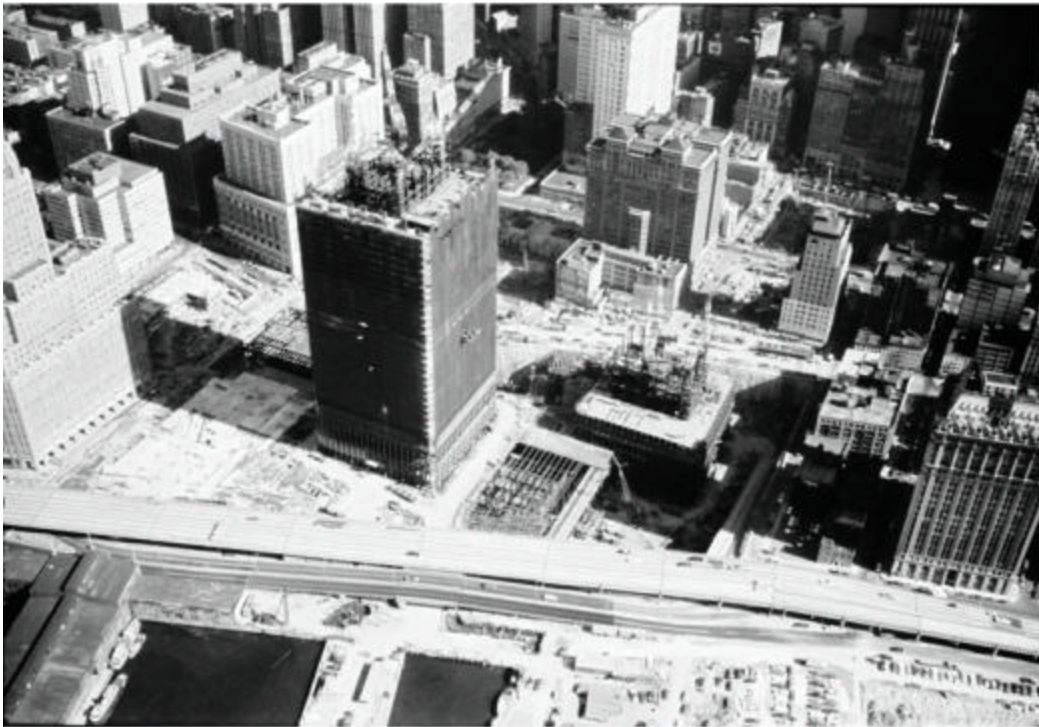
North and South towers erected with cranes, interior towers in core area supporting four cranes are shown, decking
