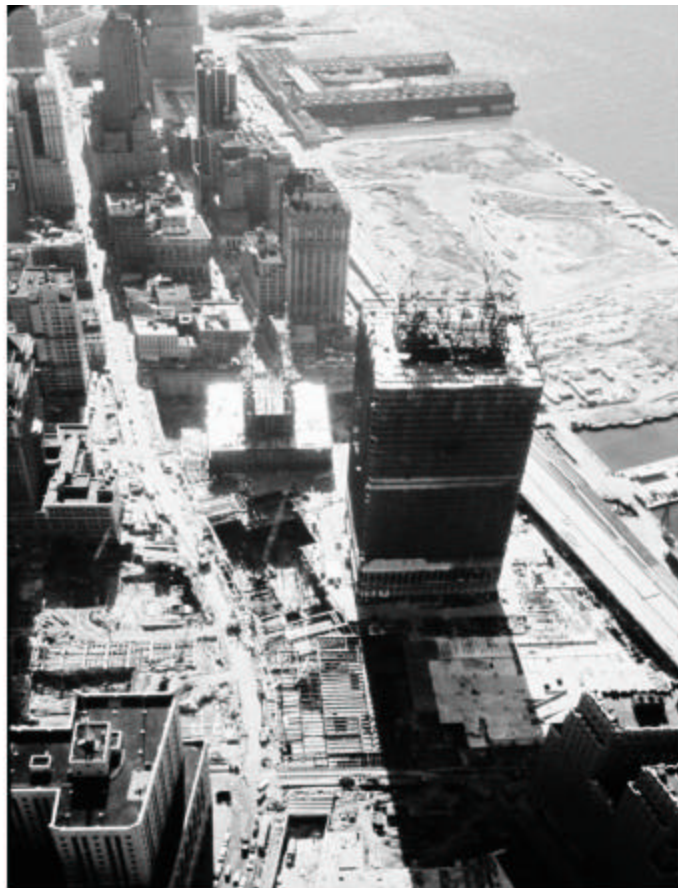
North and South towers, Land Fill area, partial demolition completed East of Greenwich Street, (BMT tunnel not exposed)
