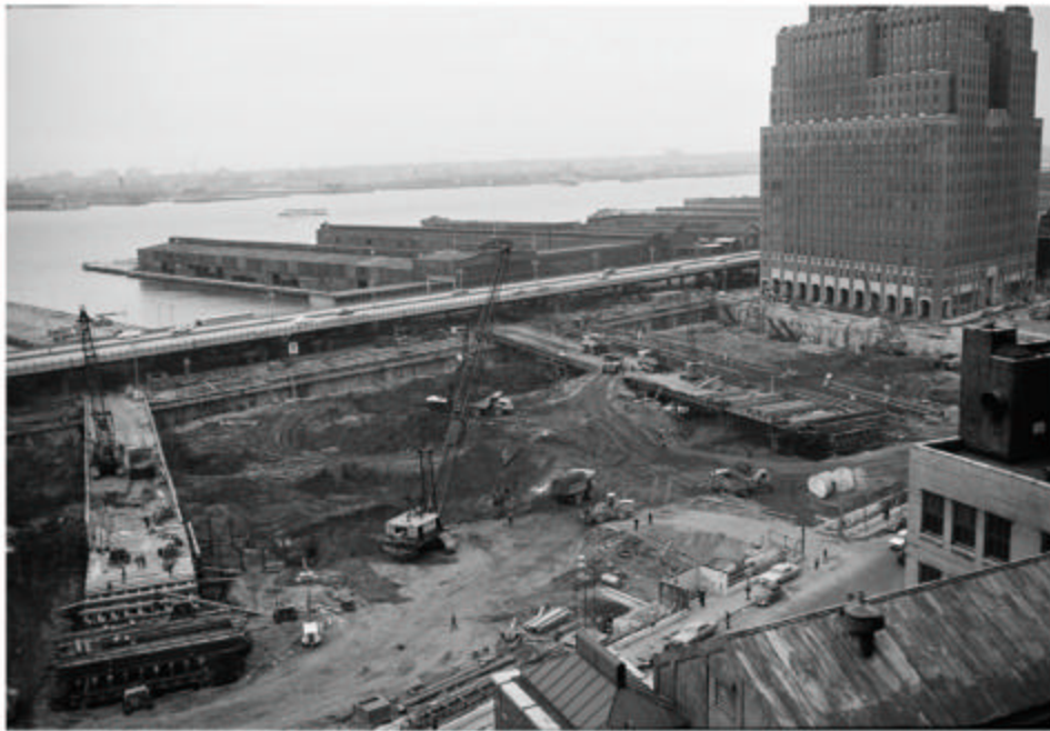
Basement excavation, construction bridges under construction, berms & earth slopes, north PATH tube supported
