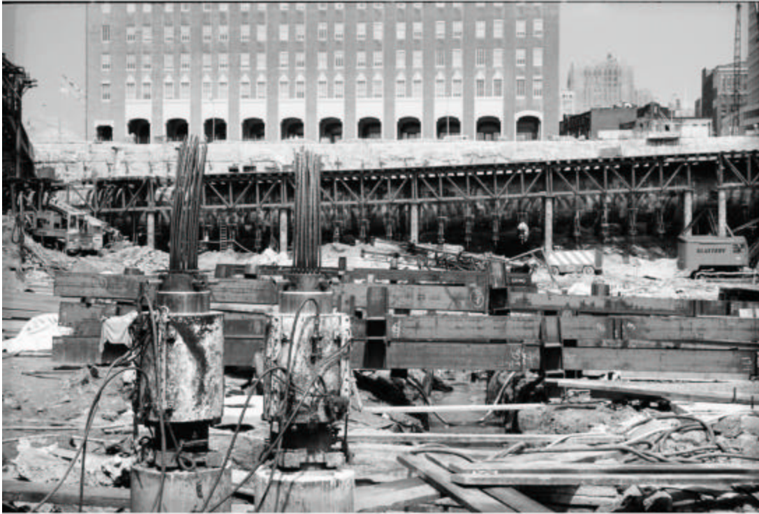
Load Cells utilized for full scale footing load test on Manhattan Schist Rock, ( E = 200,000\text{psi} , 1/100 of intact rock)
