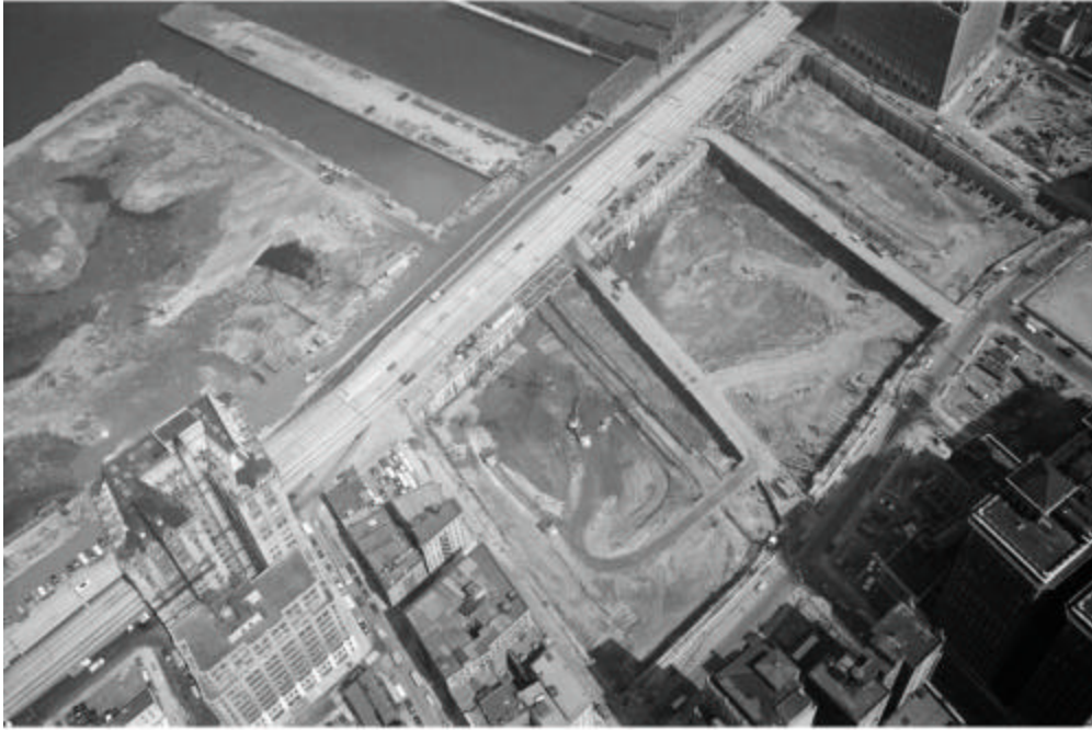
Basement excavation, both tubes exposed, considerable fill placed in Land Fill site, two interior construction bridges
