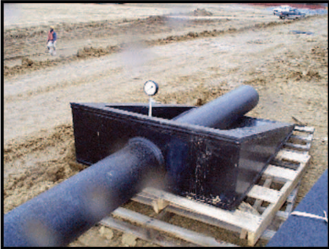
Figure 26. Penetration box delivered from the fabricator, prior to installation. The penetration box was fabricated with a chamber to allow pressure testing of the welds. Welds were tested at the fabricator and following installation using the pressure gauge shown. Following pressure testing, the gauge was removed, and the chamber filled with bentonite pellets.
