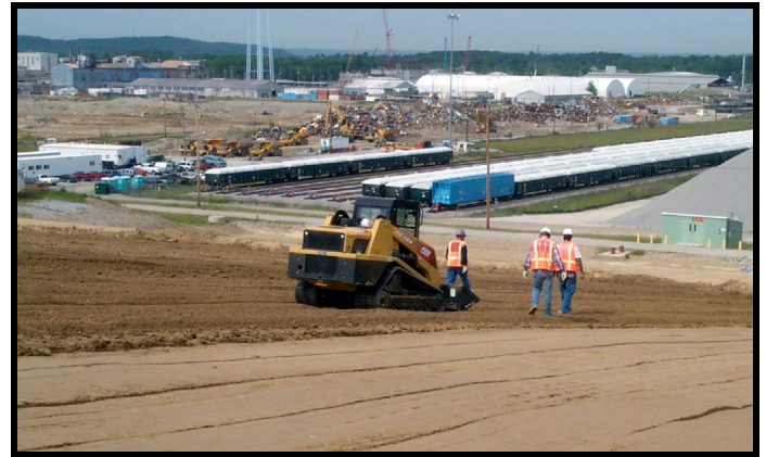
Figure 15. Construction of the final cover system CCL. The soil in the foreground is placed material that has not yet been compacted. The surface has been sealed to promote storm run-off and prevent drying. The small tracked loader holds oversized rock (>2 in.) collected by the workers.
