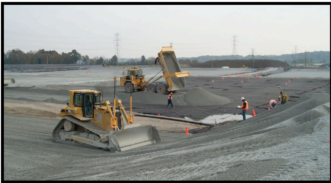
Figure 12. Placement of the LCS and LDS gravel drainage layers included the use of dump trucks operating on a 3-ft thick access road constructed from gravel and low-ground pressure dozers to spread the gravel.
