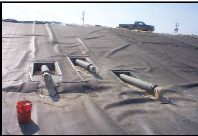
Figure 27. Liner penetration boxes installed in the secondary liner. HDPE geomembranes are welded directly to HDPE flat stock used to construct boxes.
