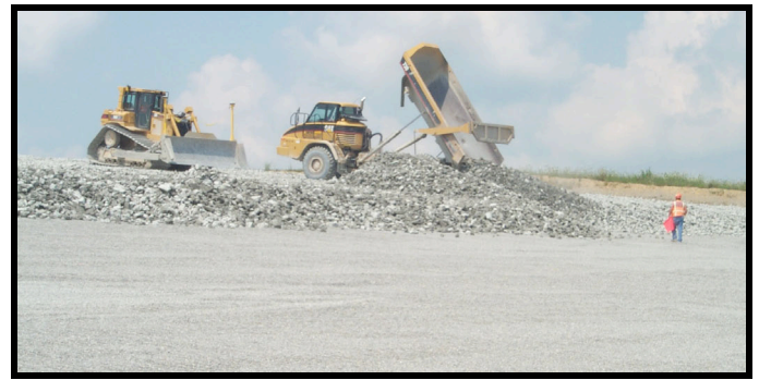
Figure 16. Placement of the 3-ft. thick biointrusion layer over the cover drainage layer.
